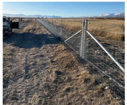
One of the break-away sections at Edwards stream. Here fence sections (x6) are designed to give way without pulling extensive lengths of fence down in the event of flood. Also, the rabbit netting is clipped to the downstream side, so that grass debris build up will hopefully sacrifice the rabbit netting only.
